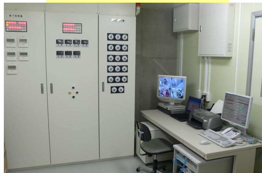
3. Monitoring & Management Room
